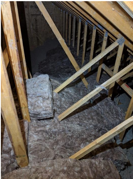
Trunk line covered with fiberglass insulation.
