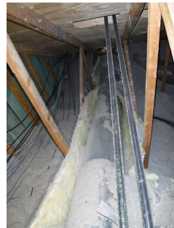
Trunk line insulation has completely fallen off.
