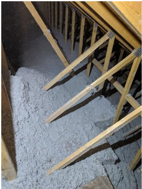
Trunk line and attic area is covered with blown-in insulation where needed.
